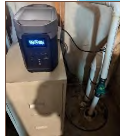
Listed Practice: Sump Pump Battery Backup
